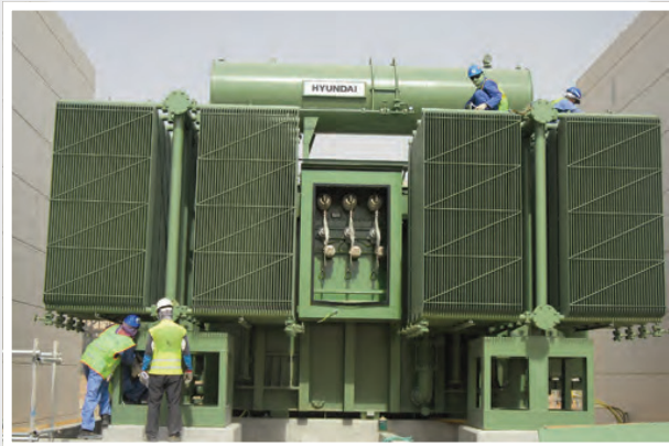
Step-Up TR, 11/230KV 40 MVA
