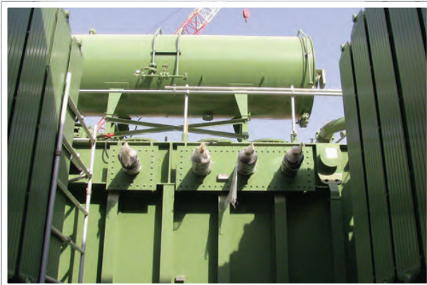
Step-Down TR, 220/33KV TR.
