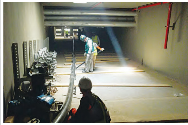
33KV Power Cable 1C-630sq
