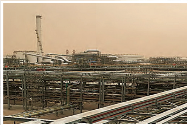
Pipe Rack for Cable Tray
