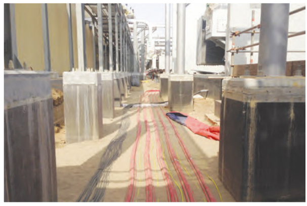
Underground MV Cable
