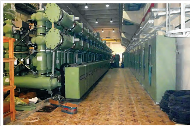
Gas Insulated SWGR Incoming Feeder 2,500A
