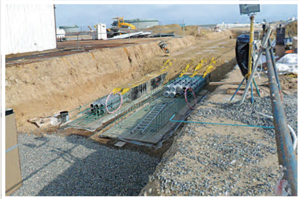
Duct Bank for HV Cable
