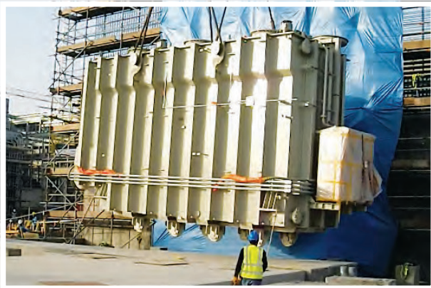
Step-up Transformer 380/13.8-18KV
