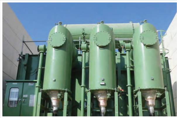
Auxiliary Transformer 13.8/6.9KV
