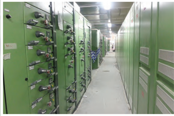
SubStation LV SWGR/MCC Room
