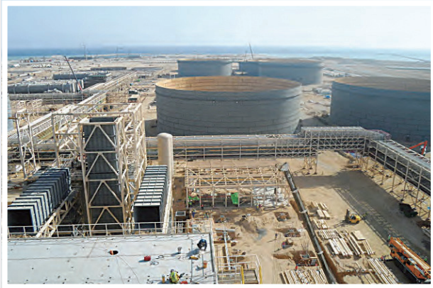
Pipe Rack For Cable Tray
