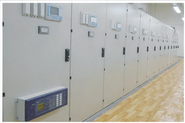
132kV SWGR Installation
