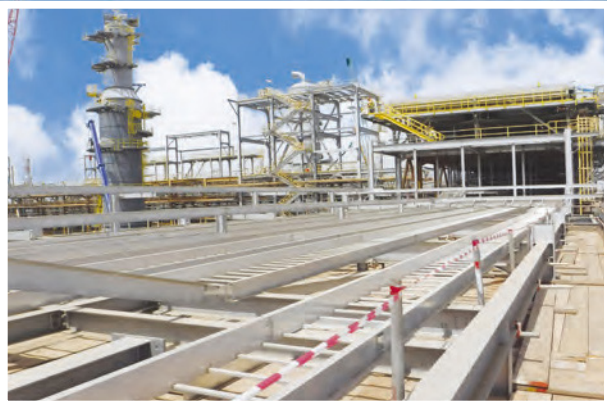
Cable Tray at Pipe Rack
