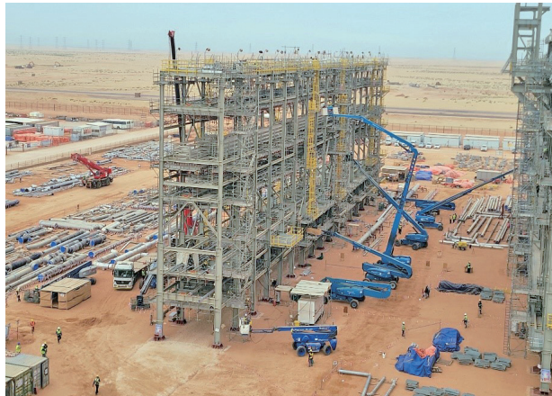
Jafurah Gas Processing Facilities Project [Saudi Arabia]
