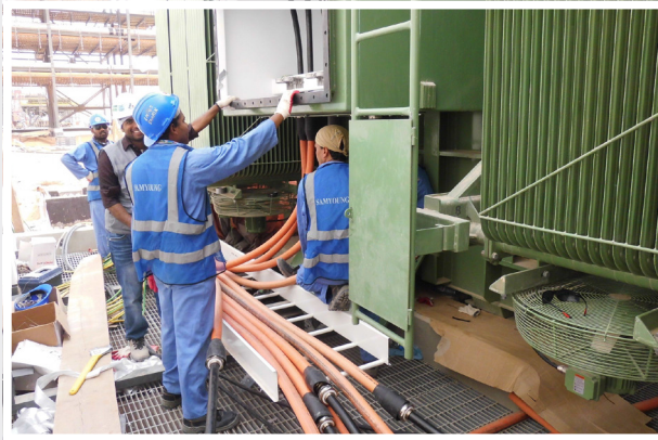
HV Cable Termination
