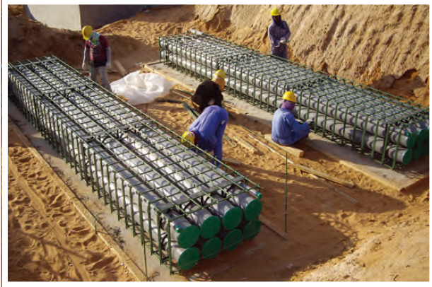
Duct Bank for HV Cable
